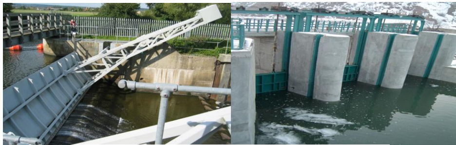
Fig. 2. Radial sluice gates and vertical sluice gates
