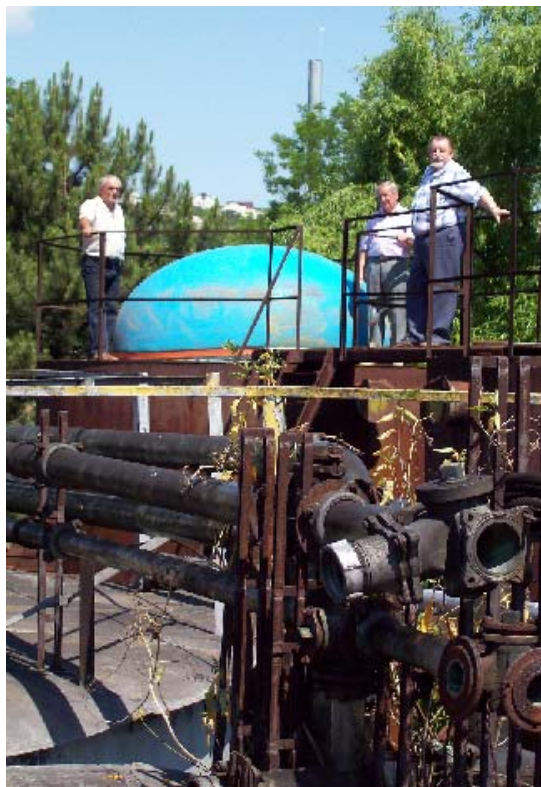
FIGURE 2. General view of the biogas reactor at Bardar Winery, Moldova
