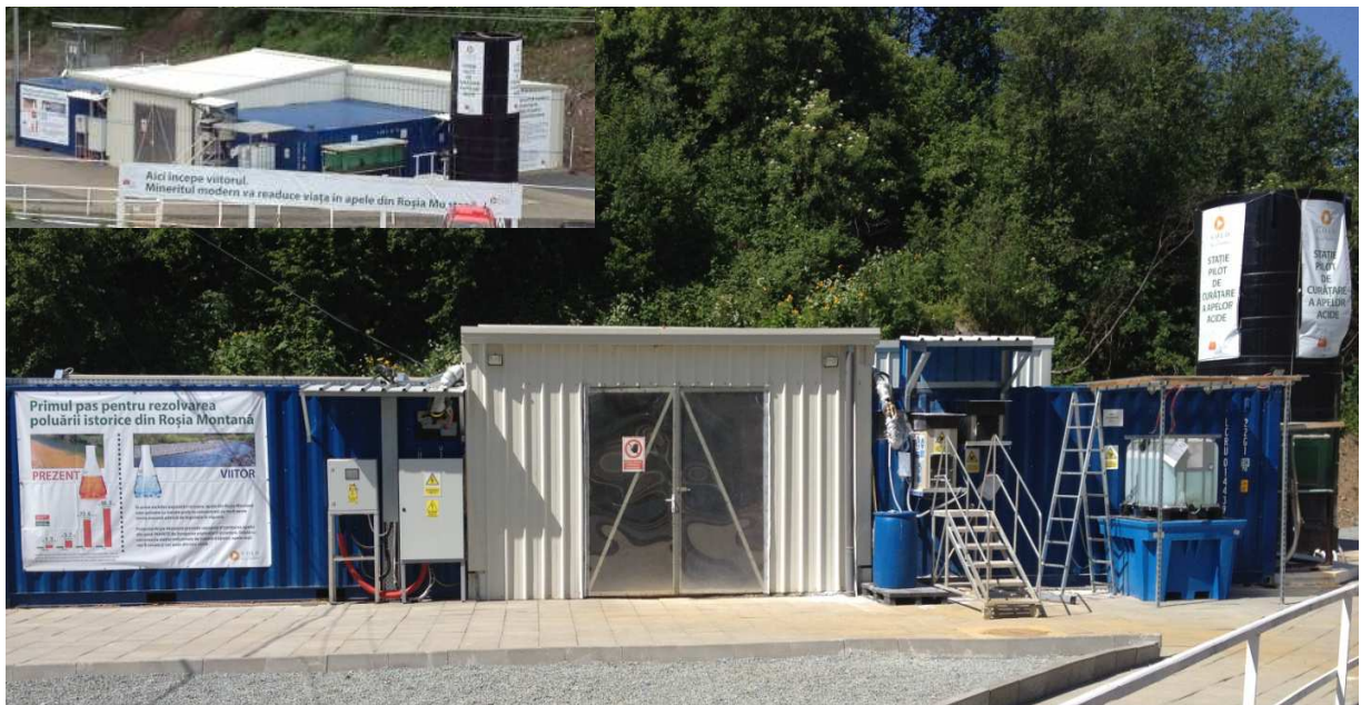
Figure 6: Overview of the Pilot Plant
